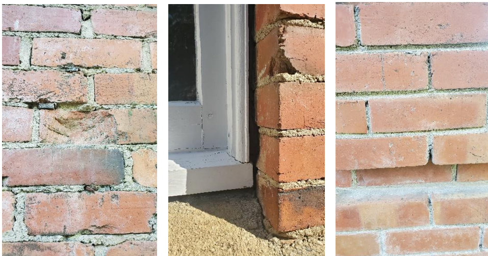
Figure 1: Rough bricks and gaps around joinery where plastering was originally anticipated.
